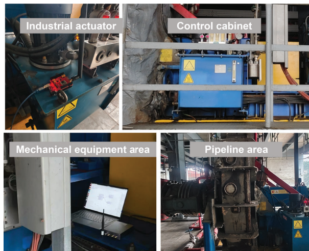
Fig. 7: Representative industrial deployment environments in an operational factory.
